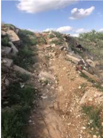
Rain damage pictured on left:
